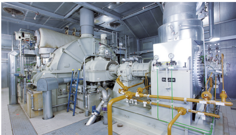
Steam turbine, lignite-fired power plant
