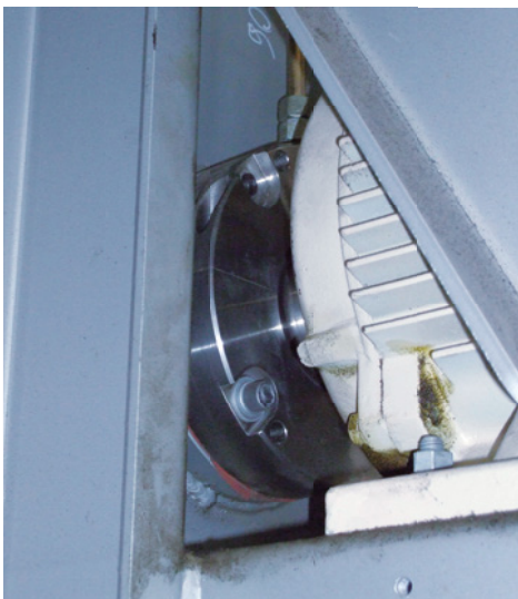
Espey WDKS-Eco, installed on a kiln housing Photo by courtesy of Aurubis AG
