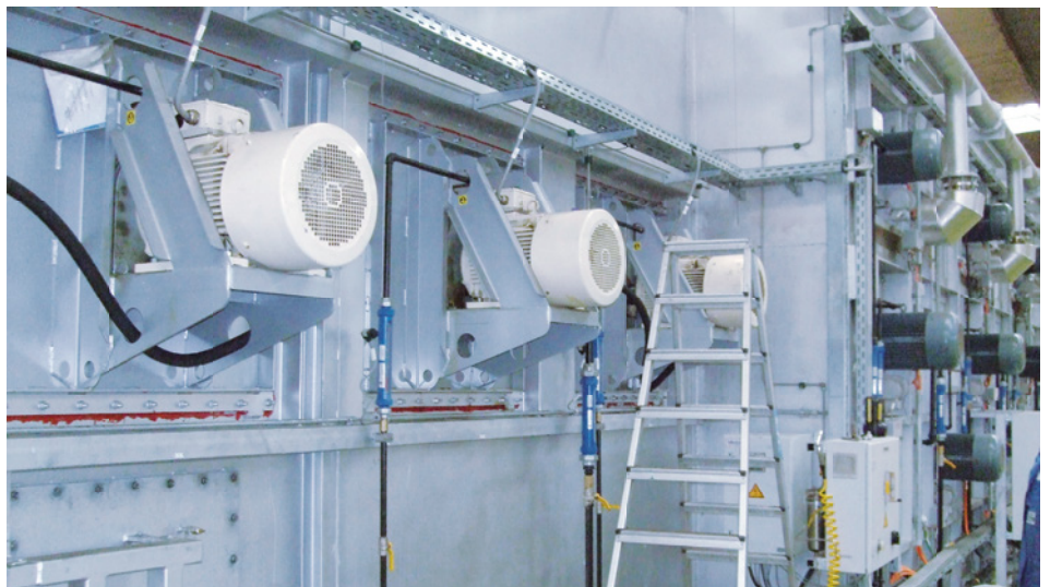
Continuous kilns' fan drives for the heat treatment of metal strips Photo by courtesy of Aurubis AG
