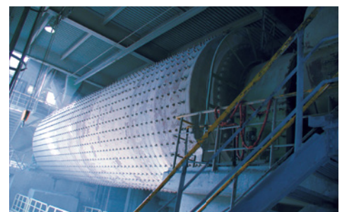
Ball mill for the cement production
