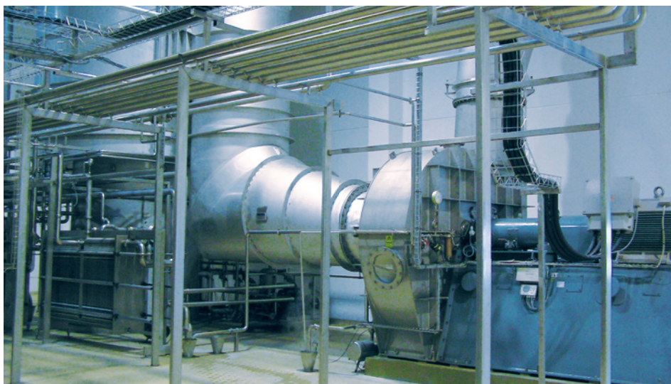
Fan installed in vapour compression plant Photo: Piller Industrieventilatoren GmbH
